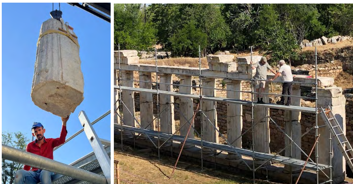
Figure 54 A-B: Sebasteion North Building. A: Re-setting column. B: East end of North Building scaffolded (2024).
