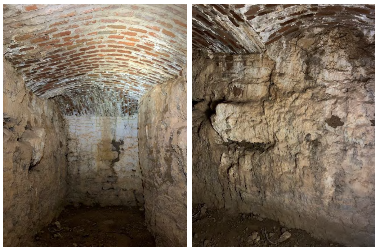
Figure 14 A–B: House of Kybele. Views into tunnel spaces (Room 25), brick-vaulted, with cave-like wall finishing, running around Room 12 (2024).
