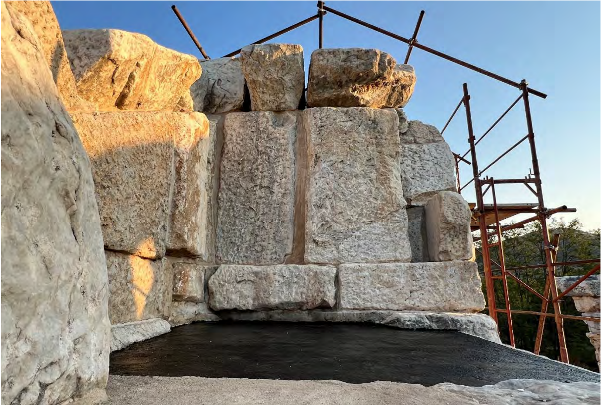
Figure 48: Tetrapylon. West side. Sealed joints and insulation with ISONEM BE 89 behind northern part of facade, above cornice level, looking north (2024).
