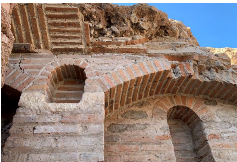
Figure 12: House of Kybele. HoK 24.2, Room 12, north wall, detail showing brickwork, niches, and springing of vault (2024).
