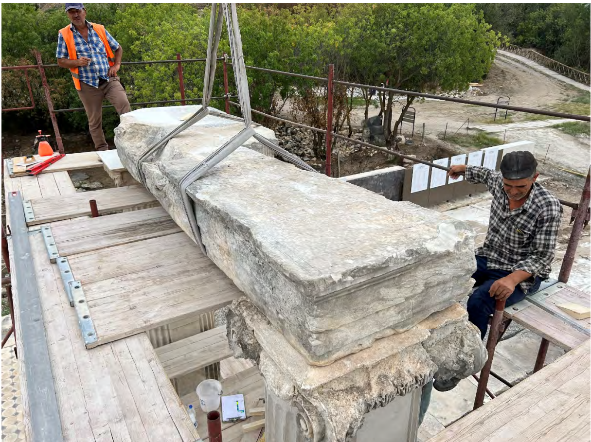
Figure 11: Civil Basilica. Placing of newly-dowelled four-metre-long architrave in original position on columns (2022).
