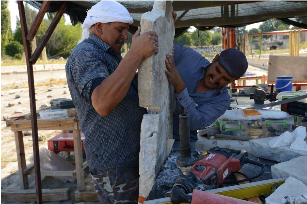
Figure 21: South Agora / Place of Palms. Conservation of foot slab from pool perimeter (2019).
