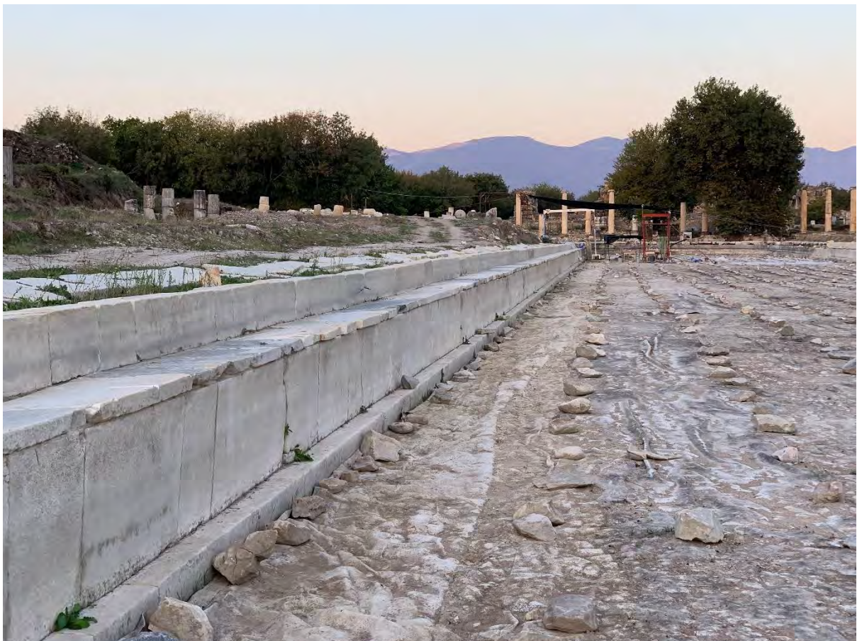
Figure 24: South Agora / Place of Palms. South side of pool perimeter after conservation (2019).
