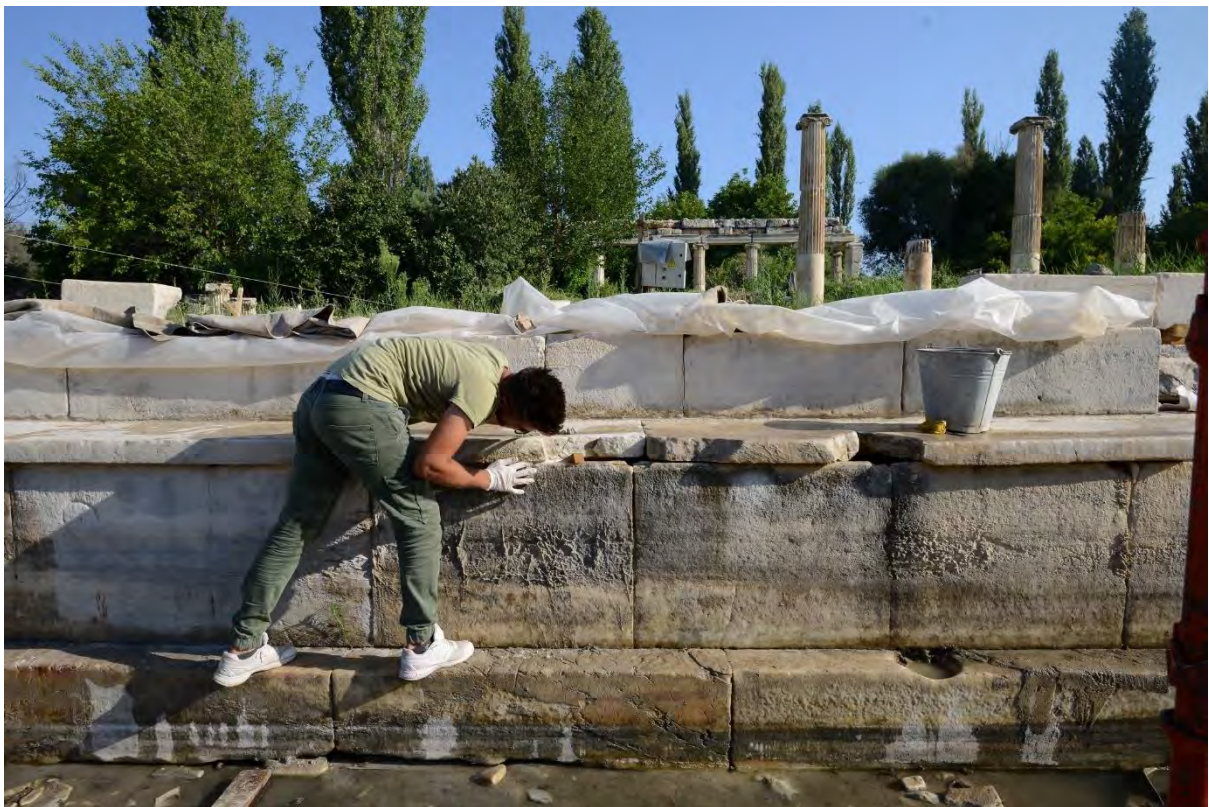
Figure 22: South Agora / Place of Palms. Conservation of orthostates of pool perimeter, north side (2019).
