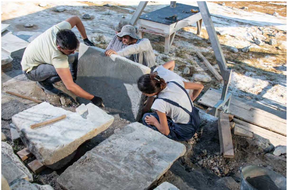
Fig. 44: South Agora – Place of Palms. Moving and repair of foot-plate slab from inner side of pool perimeter (2018).
