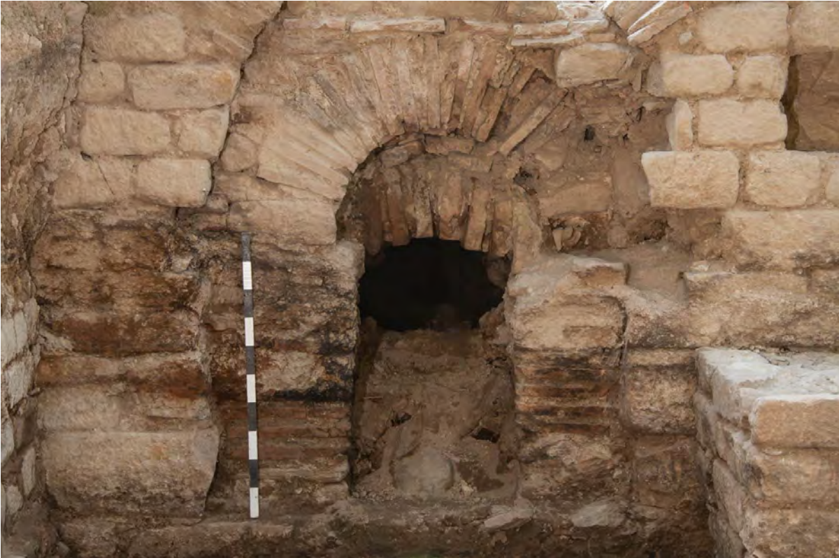
Fig. 22: Tetrapylon Street. Late antique praefurnium aperture inserted through west street wall immediately south of Niche Building (see Fig. 21) (2018).
