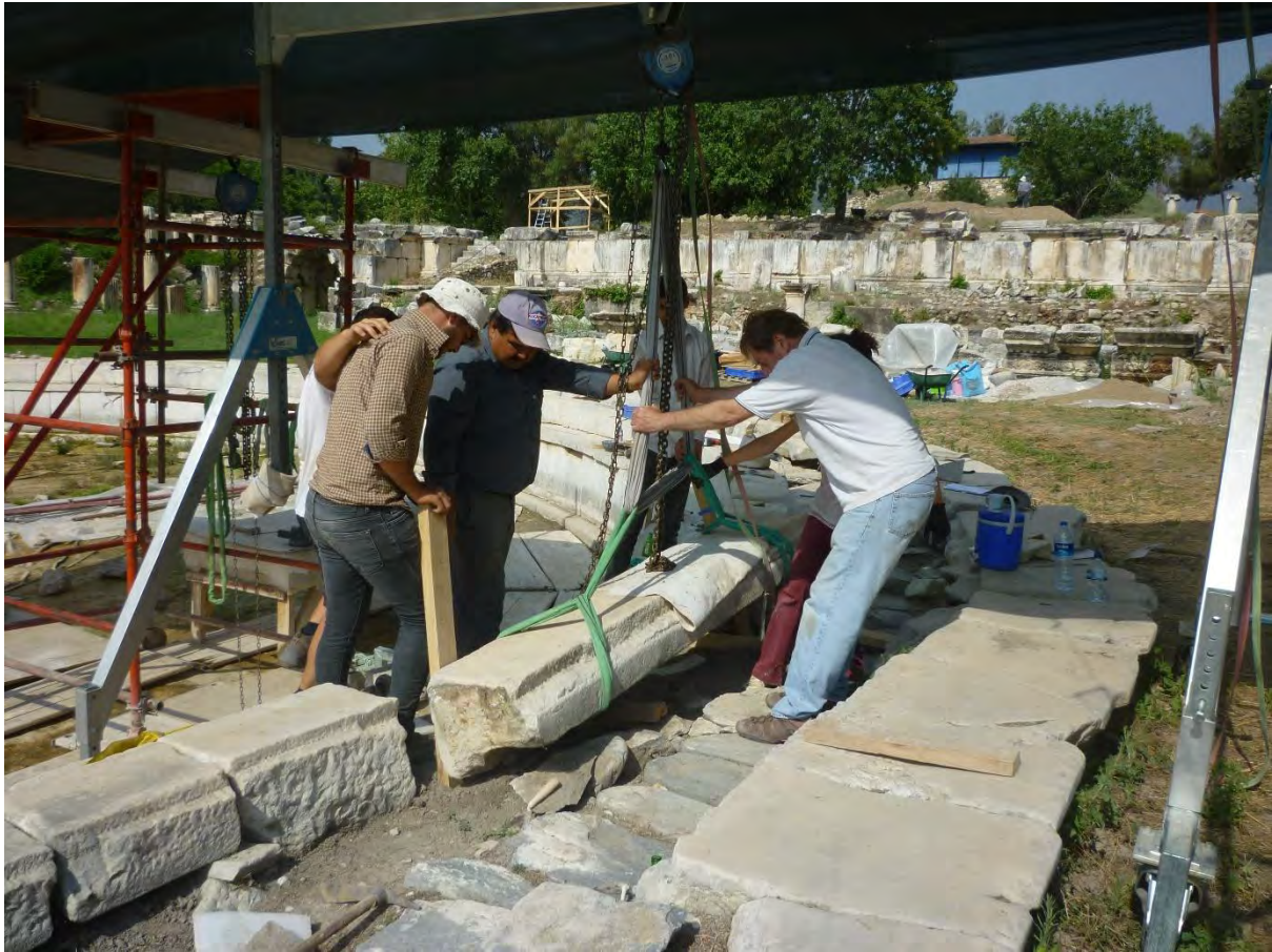
Fig. 43: South Agora – Place of Palms. Moving and repair of seat blocks from inner side of pool perimeter (2018).
