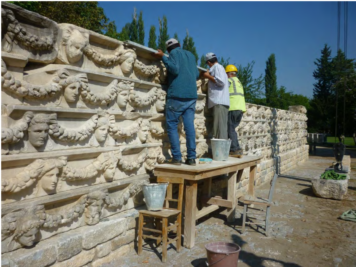
Fig. 47: Frieze Wall. Construction of wall composed of mask- and-garland frieze blocks from north stoa of South Agora – Place of Palms, excavated in 1937 and returned from Izmir to Aphrodisias in 2009 (2018).
