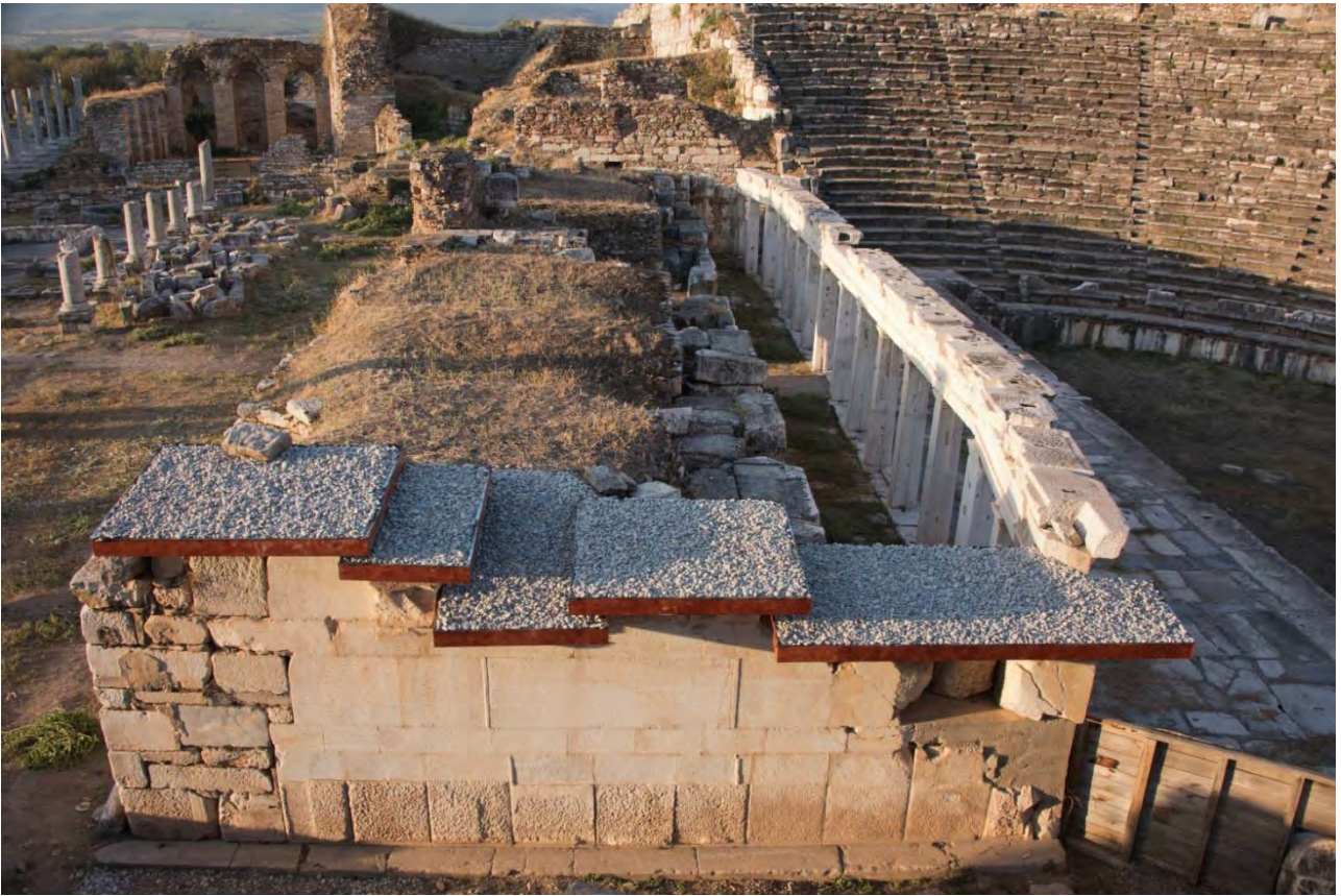
Fig. 20: Theatre, north end of stage building, new roof over inscribed Archive Wall (2016).
