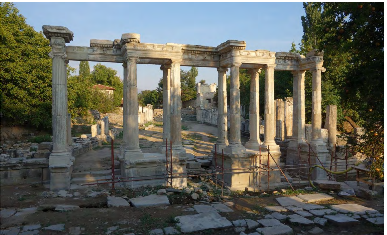
Figure 21: Sebasteion Propylon. Anastylosis: view from west, looking into Sebasteion complex from street (2015).
