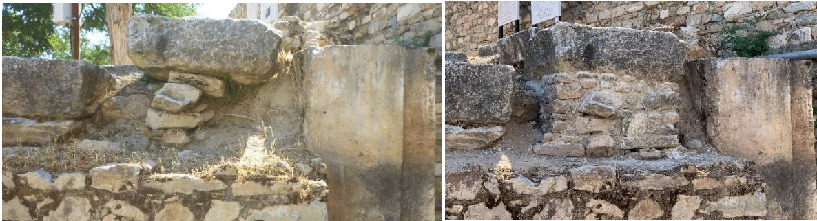
Figs. 48-49: Sebasteion Temple. Southwest angle of temple podium, showing foundations undermined (left), repaired (right) (2021)
